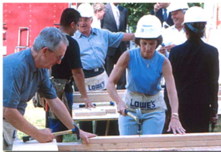
NAR President-Elect Martin Edwards and First Vice President Cathy Whatley put hammers to use at the groundbreaking on July 10 for this year's NAR Habitat for Humanity home, under construction at 1031 W. 20th Place in Chicago. The home is to be completed by November.
